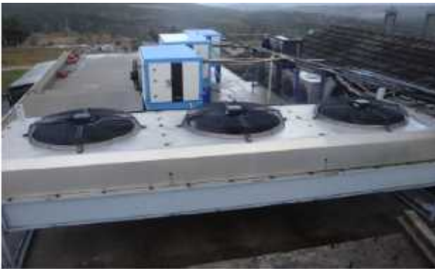
Fig. 1. Condensation groups in close proximity.
